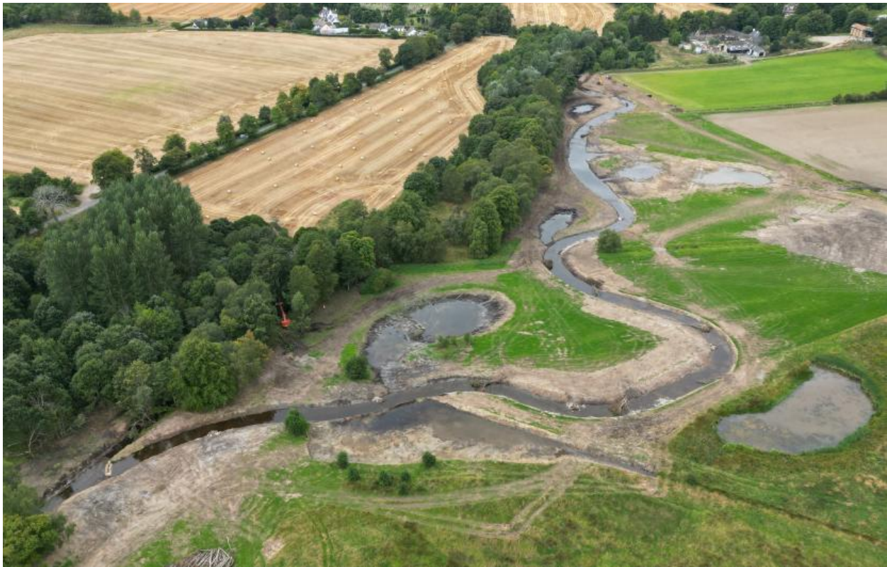
Figure 6. Aerial image of the River Peffery after re-meandering. Source: NatureScot, 2024 (credit CR Contracting Ltd.).
